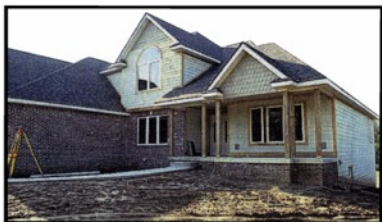
▲ Pierson-Gibbs Homes Inc. built the "shell" of the Bastianellis' house; the couple did a lot of the work.
